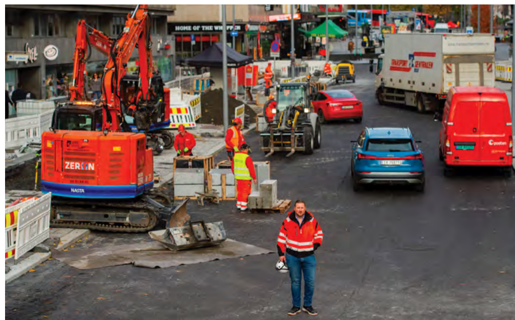
Clean construction works at Olav Vs gate in Oslo, Norway. (Image: C40/Frederik Varfjell)
