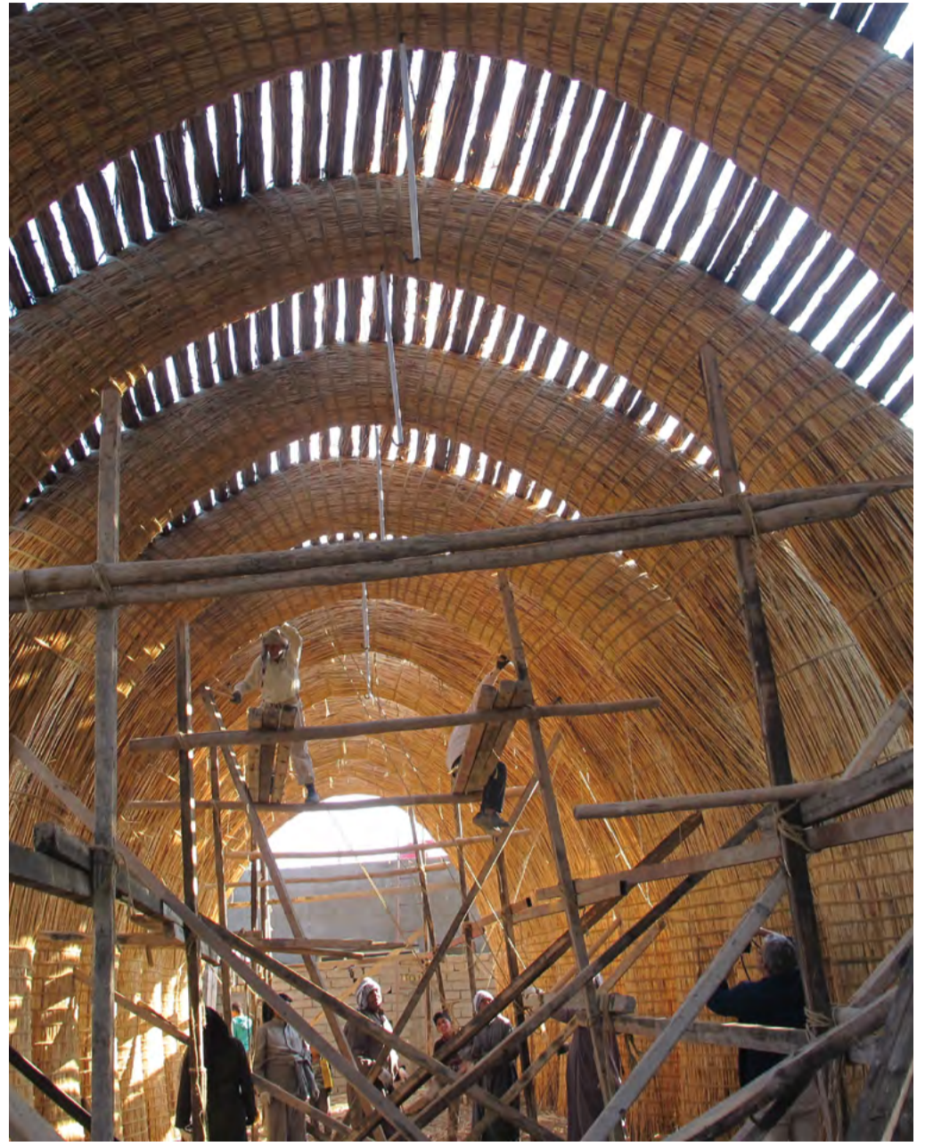
A Ma’dan house (mudhif) in the southern wetlands of Iraq, built of qasab reed without using mortar or nails, can be taken down and re-erected in a day.
