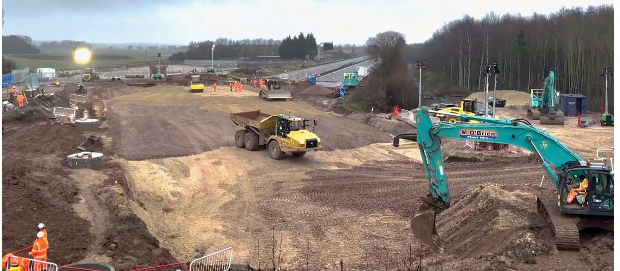
UK's first 'box slide' bridge - Marston Box M42 - preparation work. (Image: hs2.org.uk)
