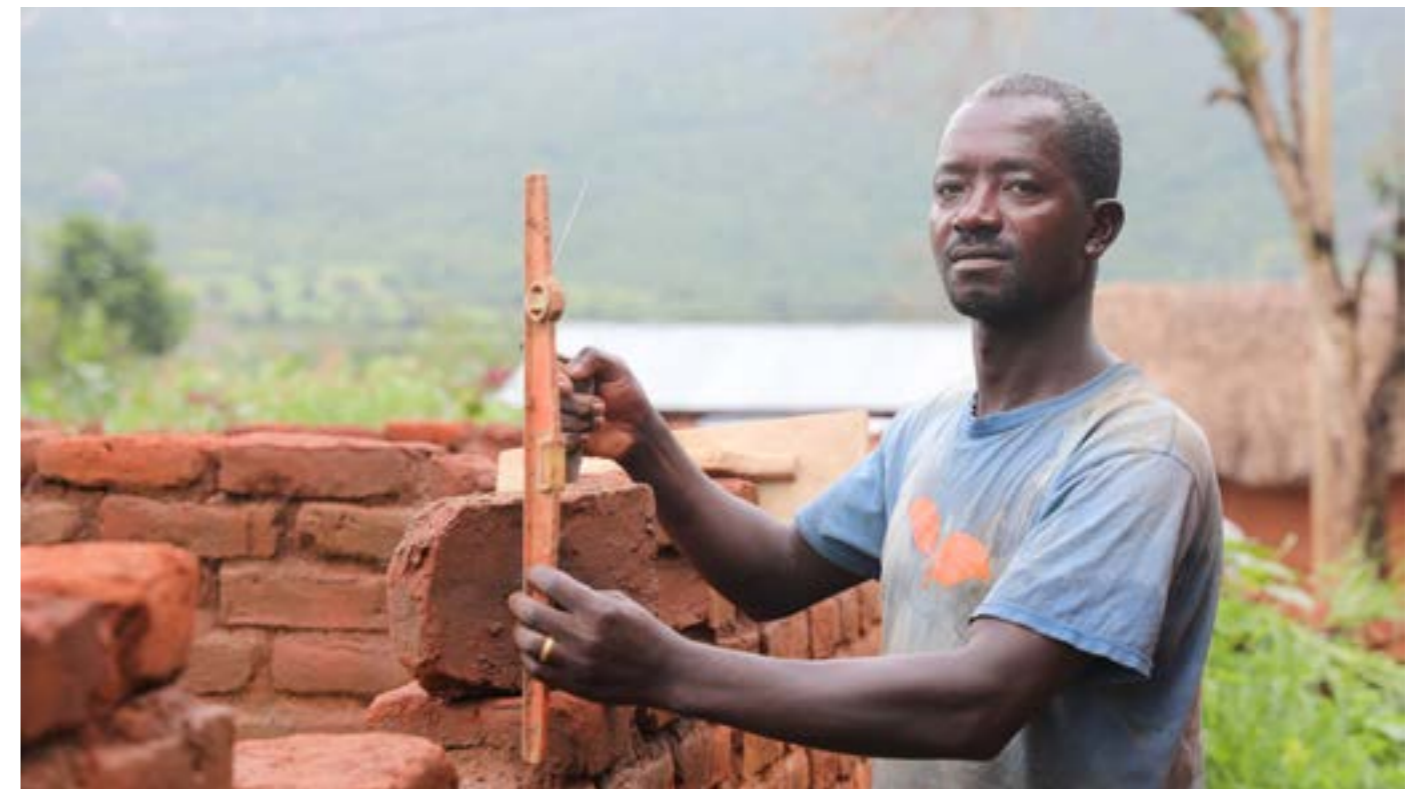
Ibumu Village, Ibumu Ward, Iringa – Babeli Kikoti works on the wall of an incomplete building. Apart from being a PLHIV Peer Educator and TB Community Health Worker, Babeli is also a mason. ©USAID Boresha Afya – Southern Zone/Mhando.
