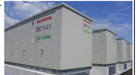
【Examples of Large-Scale BESS Installations in Japan】
