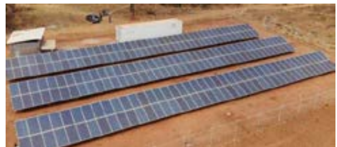
Image: Sitolo Solar Minigrid (Source: Community Energy Malawi)
