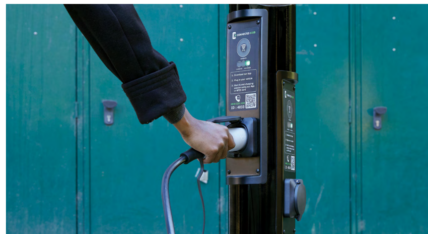
Connected Kerb charging station. (Image: Connected Kerb)
