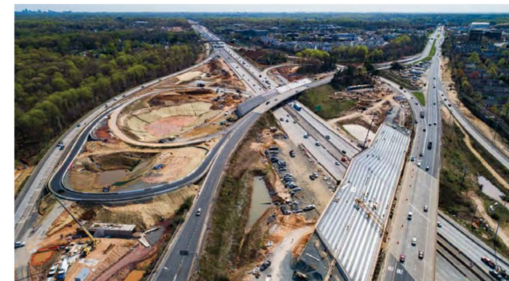
Ongoing construction at the Route 50 interchange with Interstate 66 in Fairfax, Virginia, US. (Image: EPA-EFE/Jim Lo Scalzo)
