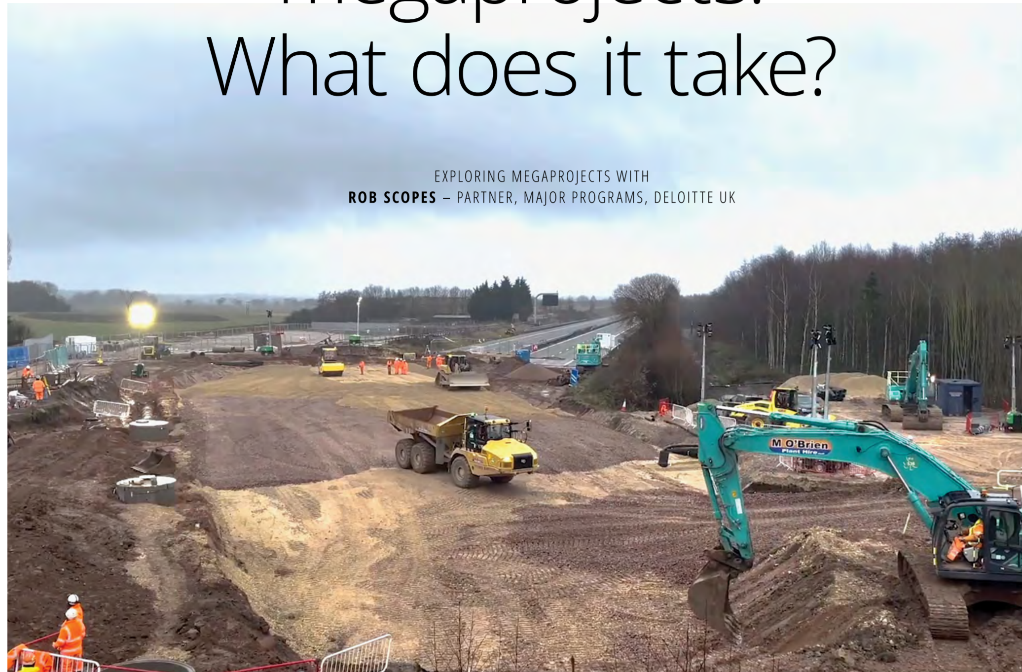
UK's first 'box slide' bridge - Marston Box M42 - preparation work. (Image: hs2.org.uk)
