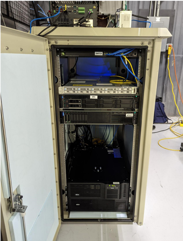
Figure 1. A single rack houses the virtualized baseband unit (CU/DU), the 4G/5G core, edge computing platform supporting smart warehouse applications, a distribution switch, and UPS. The rest of the infrastructure, including backhaul, used the warehouse operator's existing IP network.
