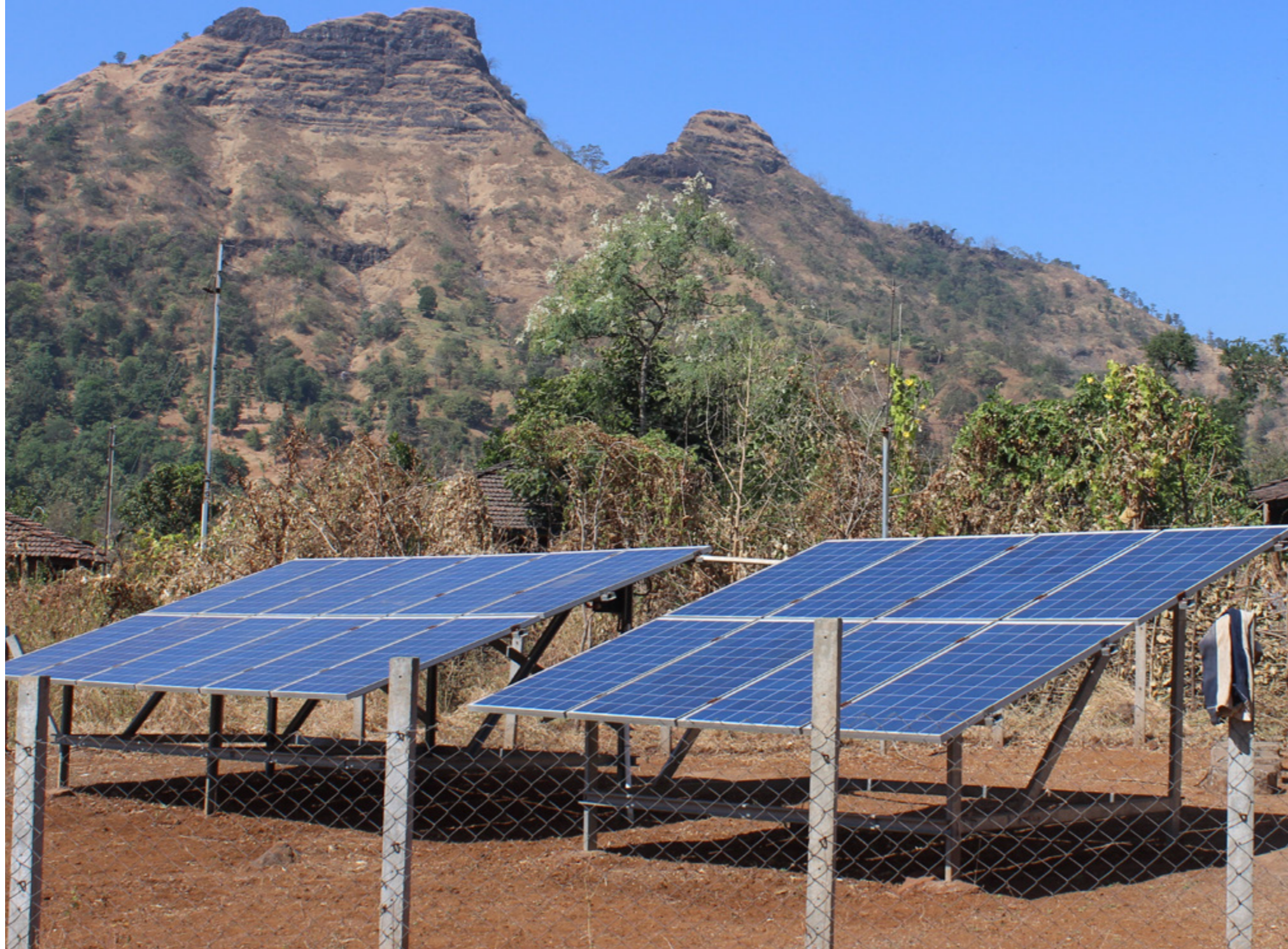
Photo courtesy : Bank of America
