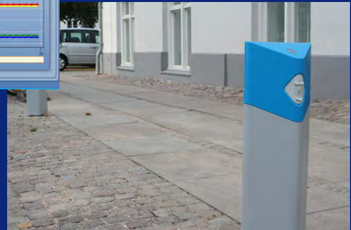
Street-side charge spots
