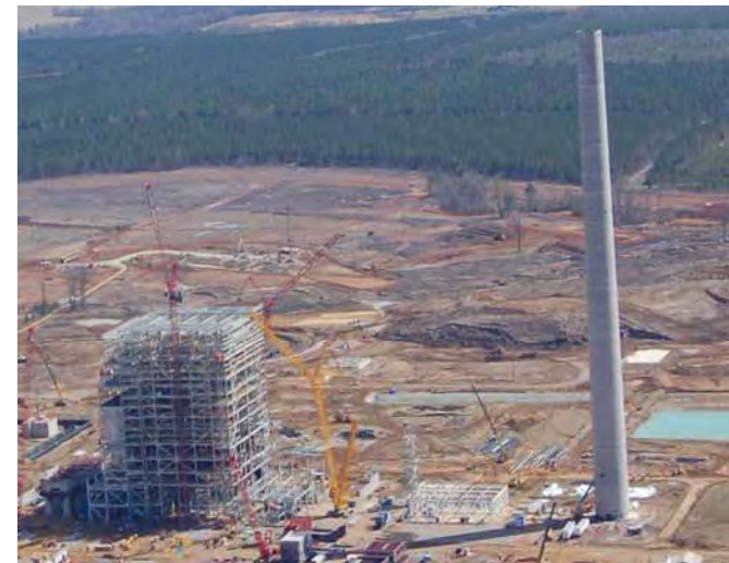
John W. Turk Jr. Ultra-Supercritical Coal Plant
